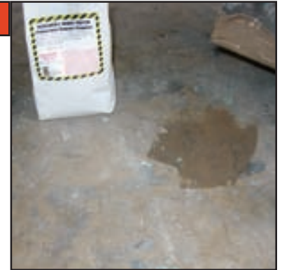
Spalled Concrete filled with DIVOT PATCH
